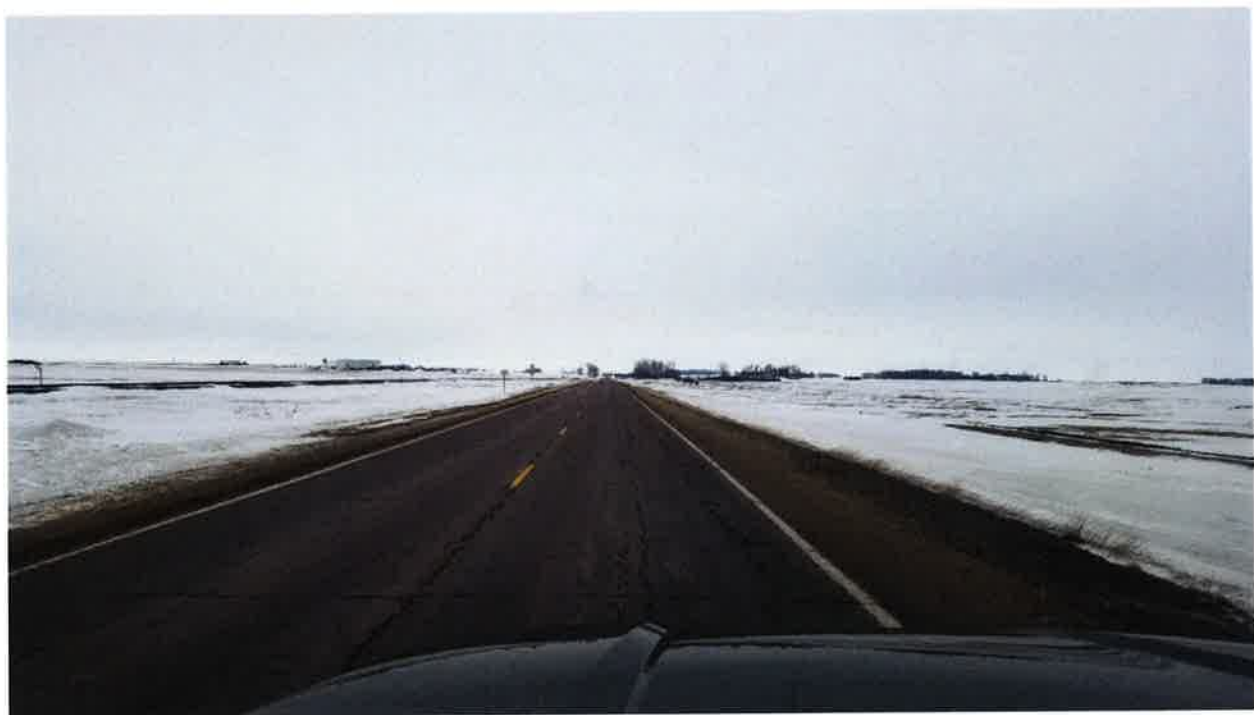
Northwest Boulevard pavement
